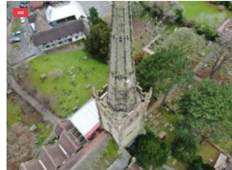
The man was suspended from the 60 metre tall steeple carrying out restoration works
