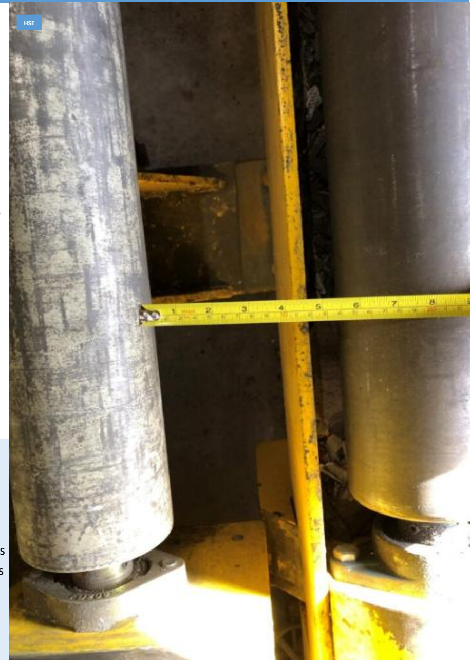
Gap in roller deck pre-accident
