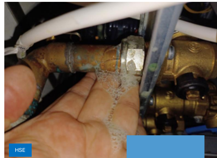
The leaking pipe
